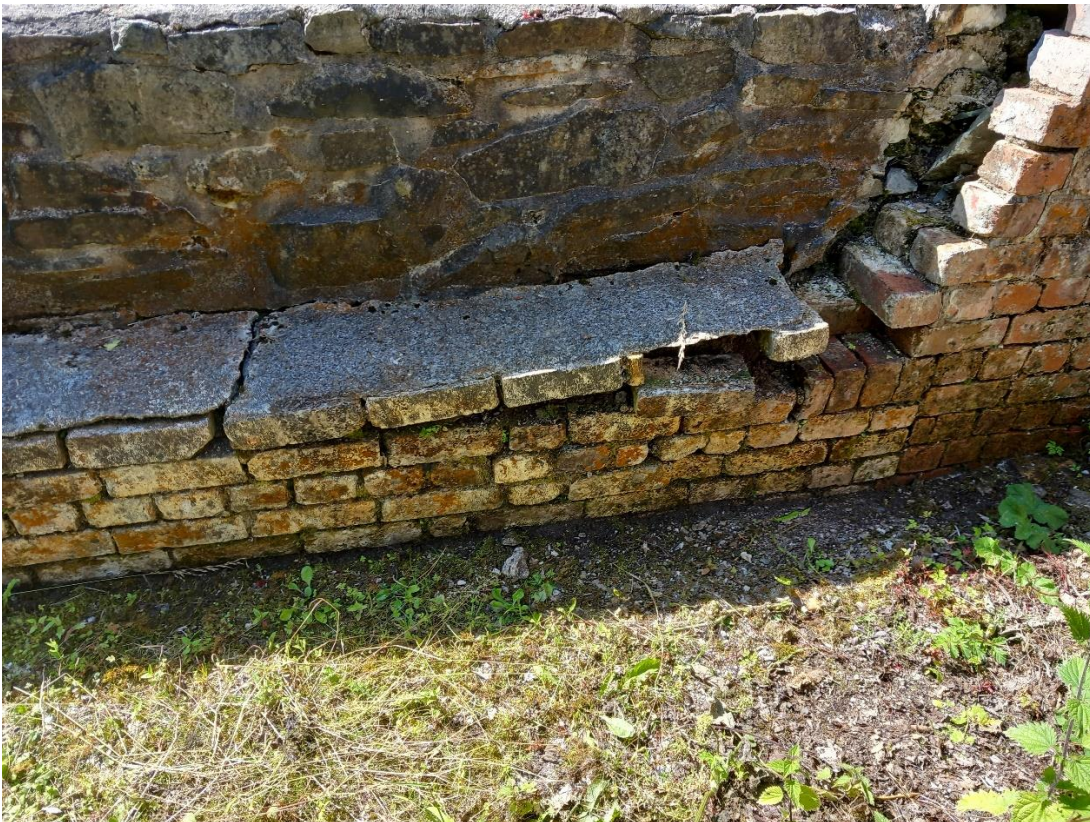
Damaged wall pre restoration
